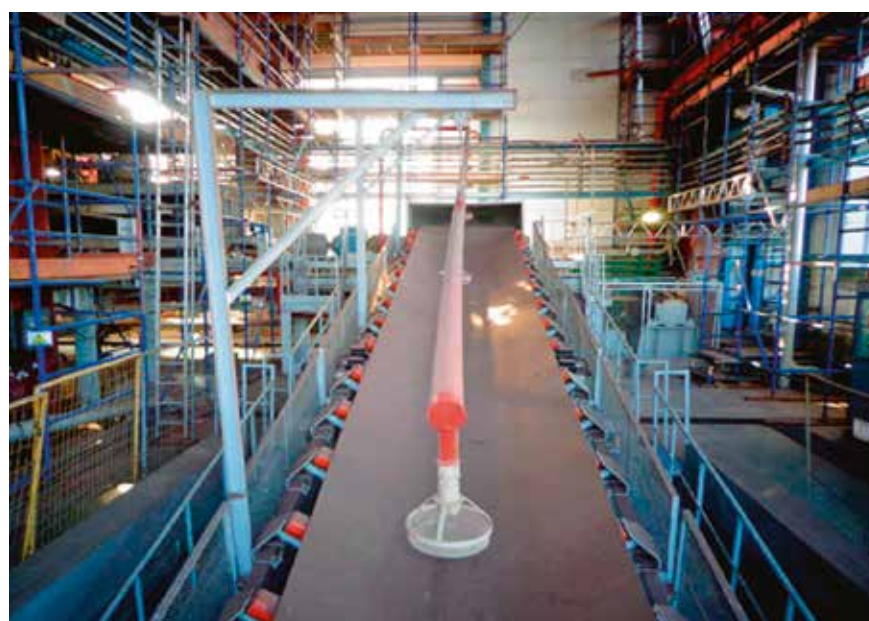
The FRS building, elev. -1,000, conveyor equipment (1/2E)
